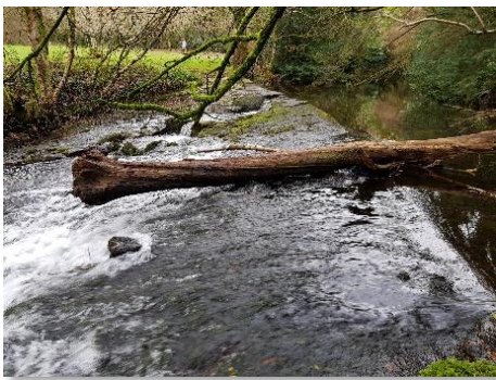
Tree trunk stuck on the weir
